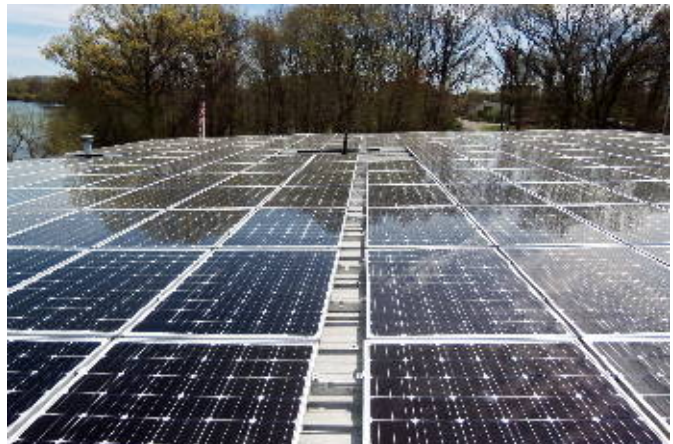
NEE installed a 210KW solar system in 2012 with over 700 panels on the facility roof. Additional upgrades include an LED Lighting conversion and a clean makeup air system.
