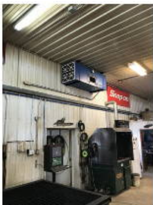
Ambient Air Cleaner in a Welding Shop
