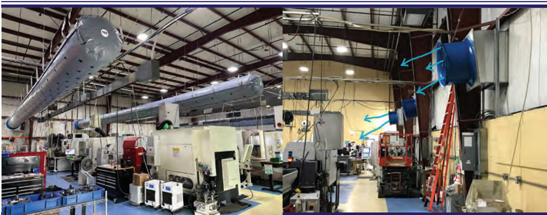
Let us design a ventilation system that will introduce and deliver fresh outside air to the employee work areas.
